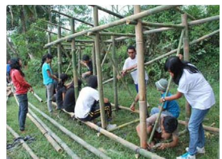
▲ Arkom's project in Mount Merapi started with the construction of temporary houses and latrines.
