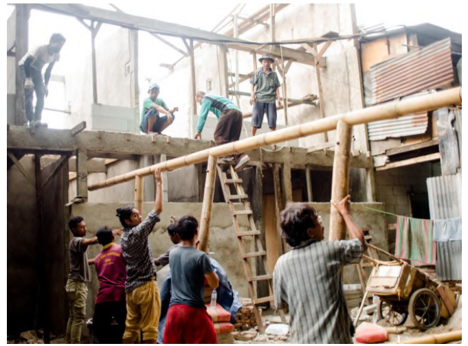
▲ The homeowners, who received training from ASF and local community builders, completed the finishing of the upper floors.
