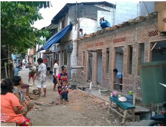
▲ A mixed team consisting of hired masons and carpenters, along with community members, constructed the ground floor and main structure.
